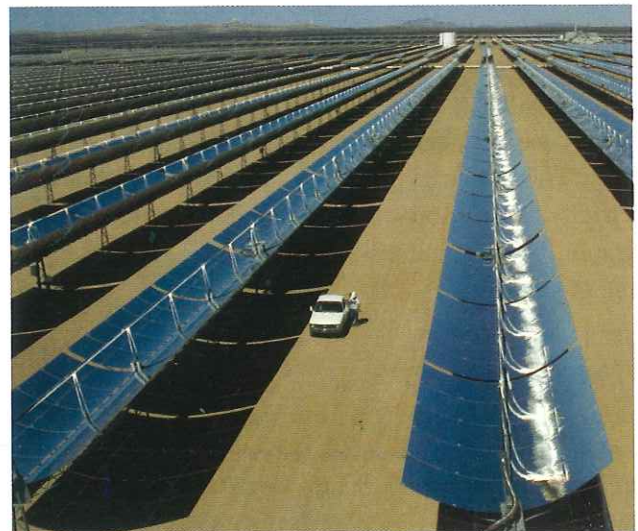
Solar energy power plant in California
